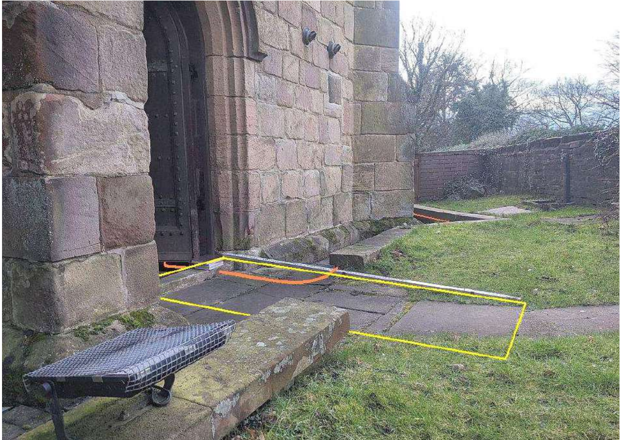
Figure 5 : Extent of new ramp, with 3-phase power cable hidden beneath
